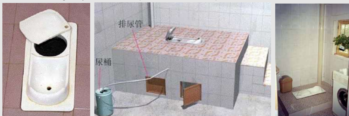
Figure 8: ecosan urine diversion squatting pan (left); ecosan in-house toilets (middle and right) (SIDA)
