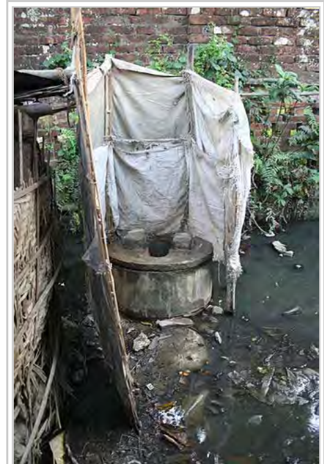
Example for lack of sanitation: Unhygienic pit latrine with ring slab in Kalibari community in Mymensingh, Bangladesh
