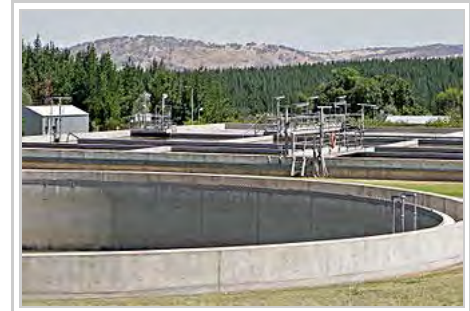
Sewage treatment plant, Australia.
