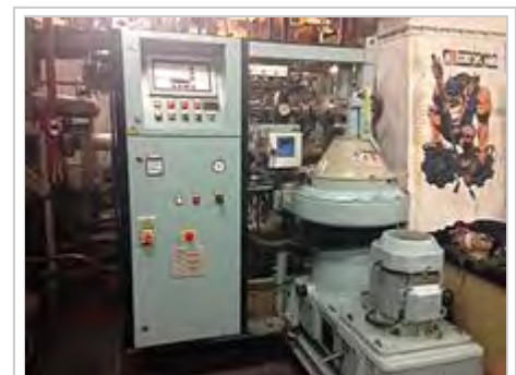
Centrifuge oily water separator
