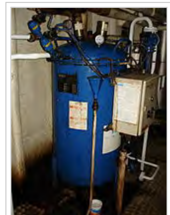
Marine oily water separator
