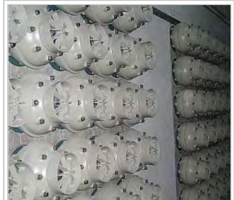
Blast protection valves installed in a bomb shelter
