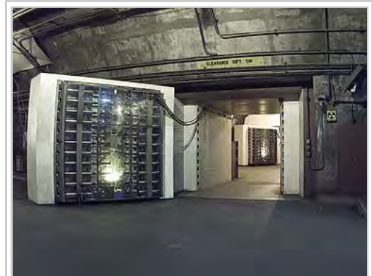
The 25-ton blast door in the Cheyenne Mountain nuclear bunker is the main entrance to another blast door (background) beyond which the side tunnel branches into access tunnels to the main chambers.
