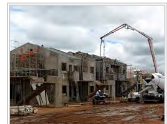
Construction of social housing in Campo Grande, Brazil using aluminum concrete formwork
