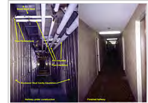
Common insulation application inside an apartment in Mississauga, Ontario
