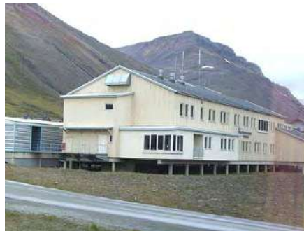
Modern buildings in permafrost zones may be built on piles to avoid permafrost-thaw foundation failure from the heat of the building.
