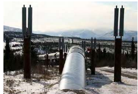
Heat pipes in vertical supports maintain a frozen bulb around portions of the Trans-Alaska Pipeline that are at risk of thawing.
