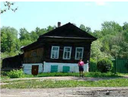
Thawed permafrost under this house caused it to settle unevenly —Tomsk, Siberia, Russia.
