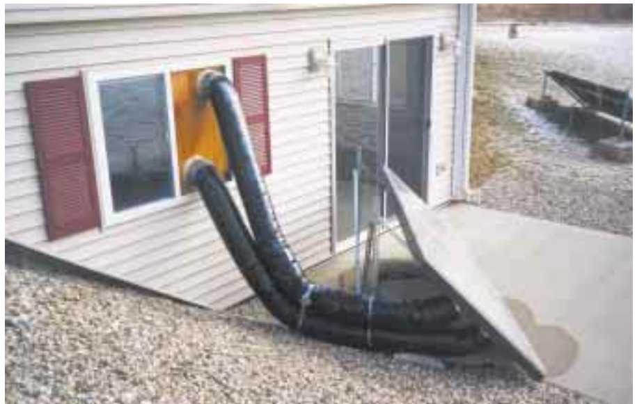
Back of the solar collector showing part of the support structure, as well as insulated cold and hot air ducts.
