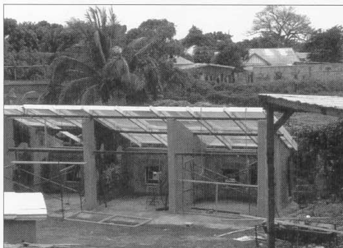
Figure 1 The solar kiln under construction, shortly before finishing installation of the glass frames
