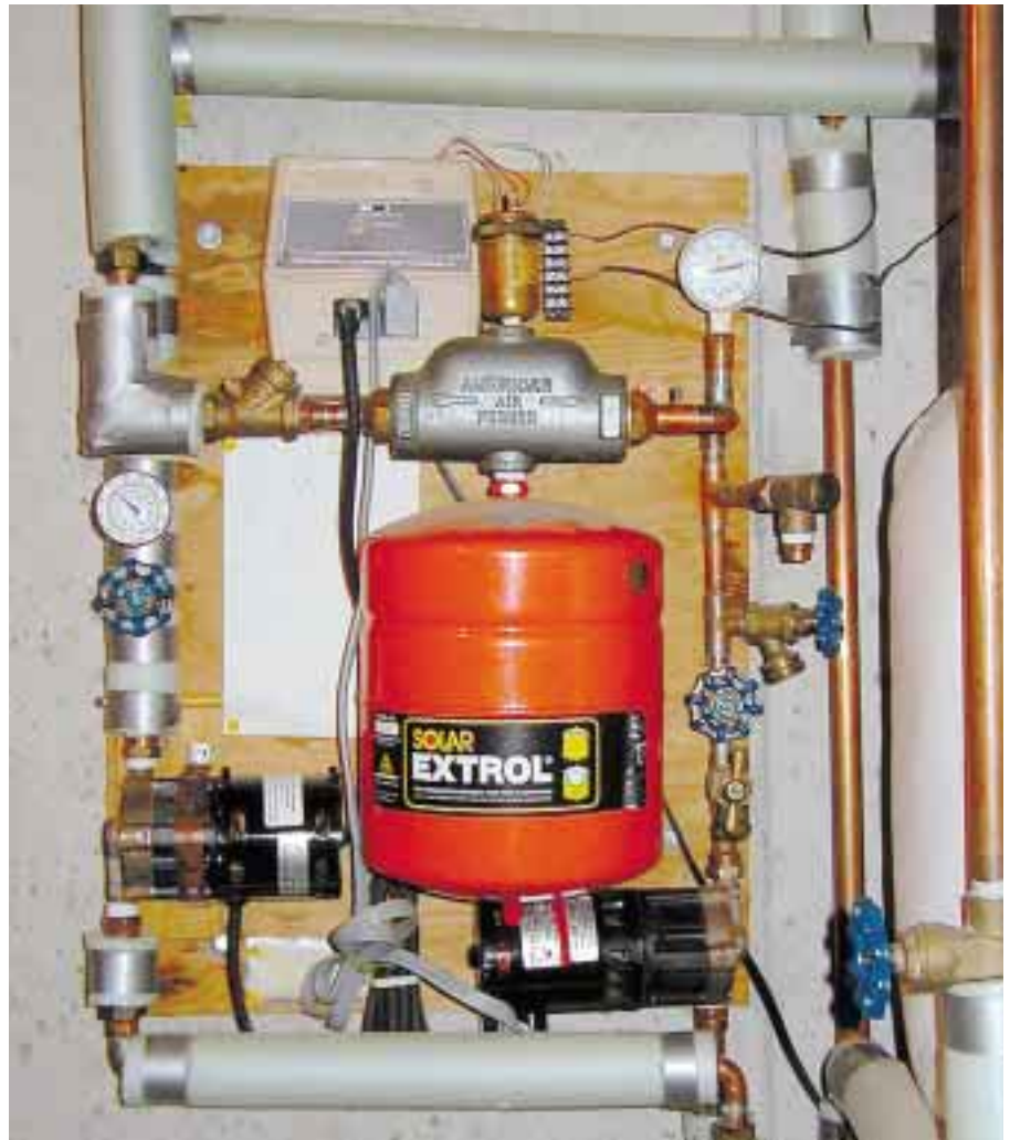
A closed loop module groups the major components on one board. This homebrew model by the author has functioned without fail since 1982.
