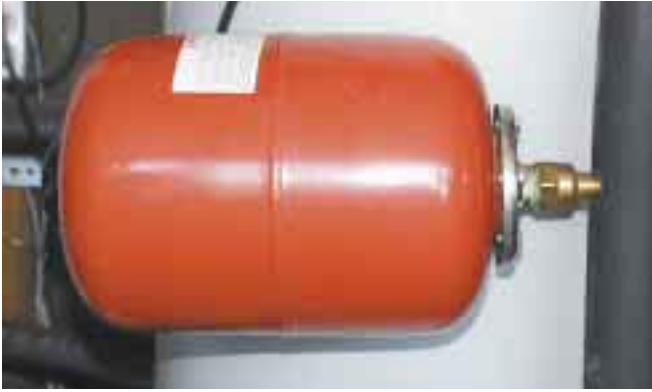
An expansion tank maintains pressure in the closed loop as system temperature changes.
