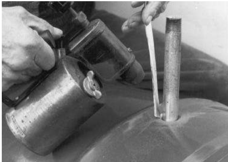
Photo 6: Then solder the piece of pipe in upright position securely into the hole.
