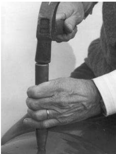
Photo 3: By using the steel cone and hammer widen one hole until a 1/2" piece of pipe fits in.
