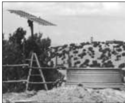
A 300-watt solar array powers a piston-type solar submersible pump located 550 feet deep in a nearby well.
