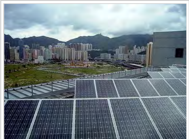
A solar photovoltaic system array on a rooftop in Hong Kong
