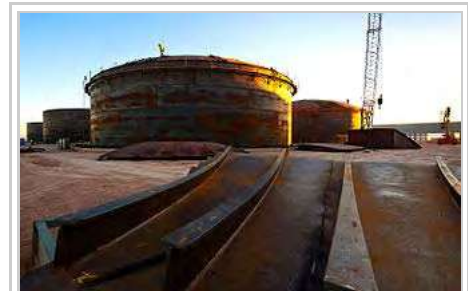
Construction of the Salt Tanks which provide efficient thermal energy storage [100] so that output can be provided after the sun goes down, and output can be scheduled to meet demand requirements. [101] The 280 MW Solana Generating Station is designed to provide six hours of energy storage. This allows the plant to generate about 38 percent of its rated capacity over the course of a year. [102]
