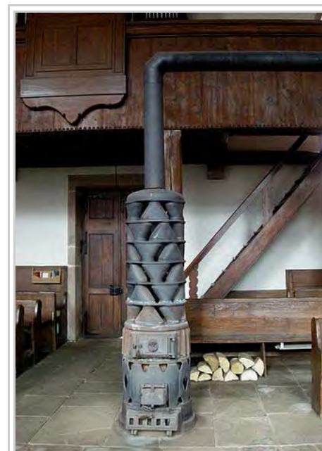
Alsatian stove with large exhaust gas heat exchanger, in Fouday church
