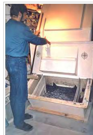
Composting container of "TerraNova" composting toilet, showing open removal chamber (town house at the ecological settlement Hamburg-Allermöhe, Germany)
