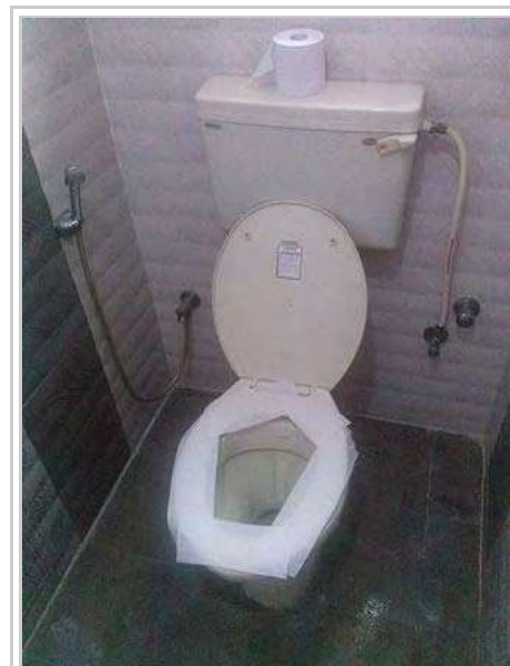
Toilet paper is also used for spreading on seat before sitting
