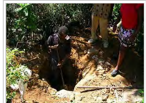
Digging the pit for an Arborloo, a type of pit toilet in Cap-Haitien, Haiti
