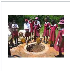
School children in Zimbabwe digging a shallow pit for an Arborloo toilet (a variation of a pit latrine), Epworth in Harare, Zimbabwe.
