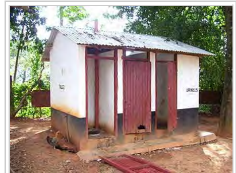
School pit latrine after maintenance has been neglected at Ambira Boys High School, Nyanza Province, Kenya
