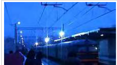
Electric arcs between the power line and pantographs of an electric train after catenary icing
