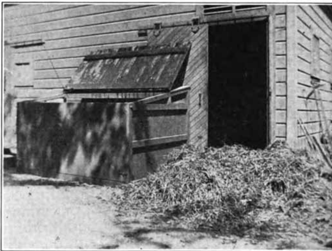
FIG. 127. — Manure bin in a position to become a fly breeding cage, instead of a fly preventative. It is suggested that the lid be permanently closed, and an opening made directly from the stable into the bin. The manure pile adjoining the bin illustrates the manner of disposal before the bin was built.
