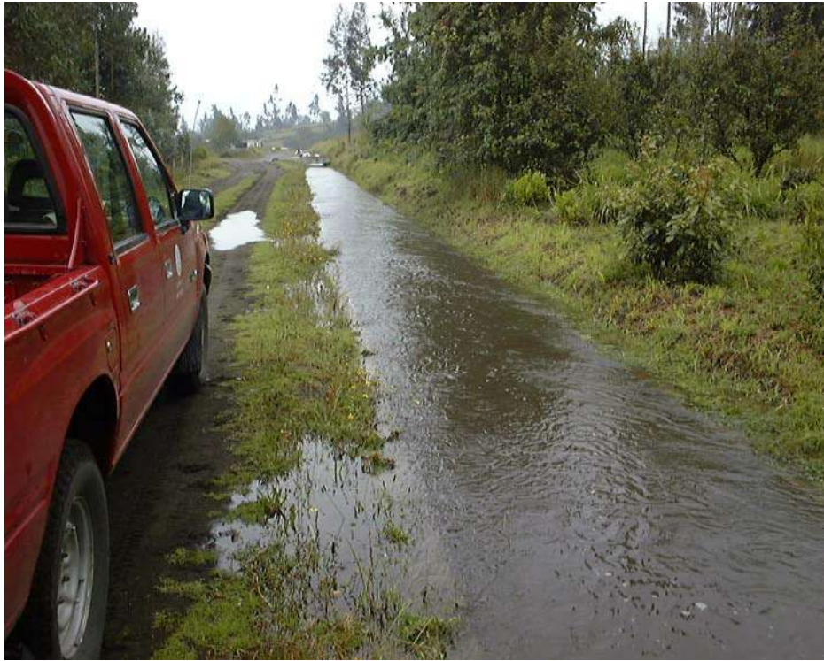
A canal which is overtopping the banks and spilling water.
