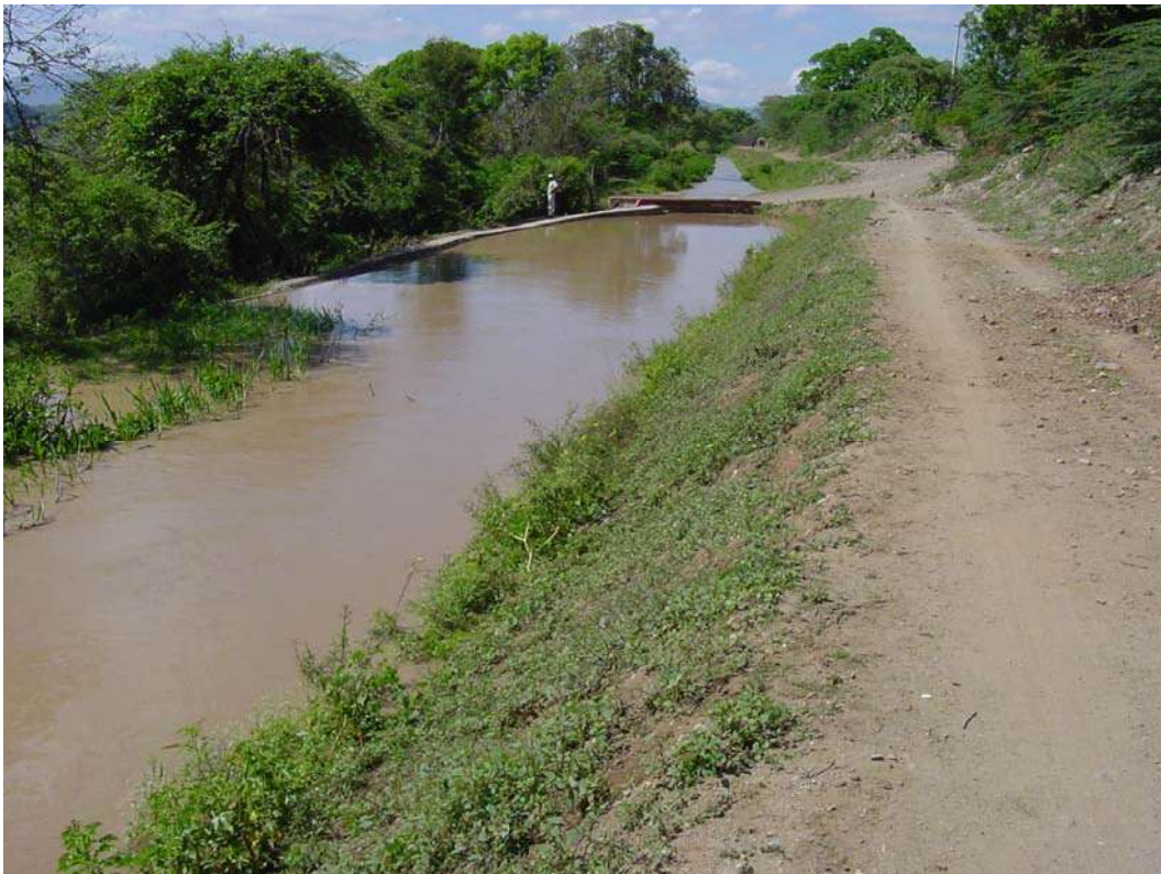
A canal with impending spillage (zero freeboard).
