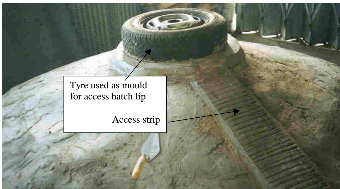
Figure 13. Showing finished access strip and old tyre used as former for access hatch lip.
