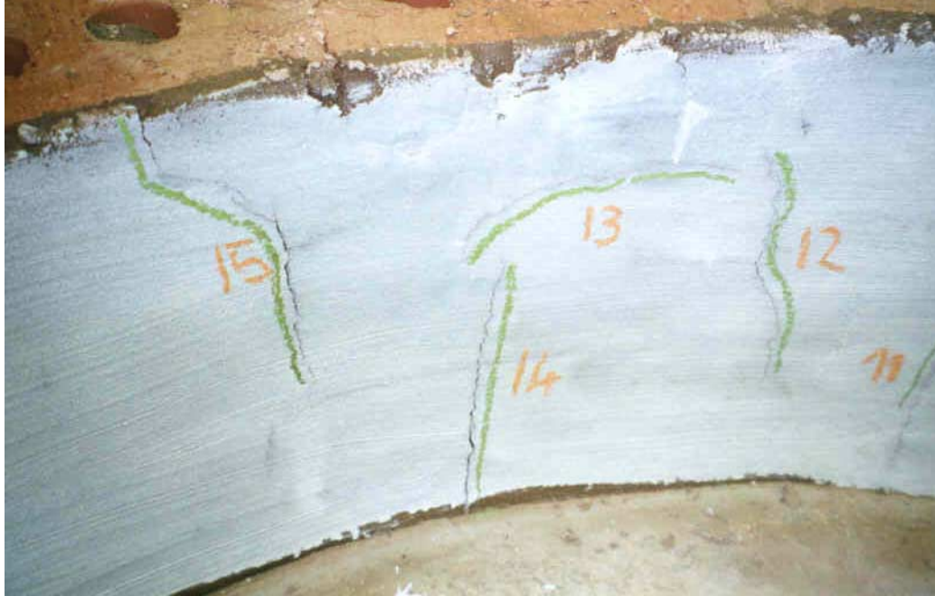
Figure 5 – Cracks in renders
