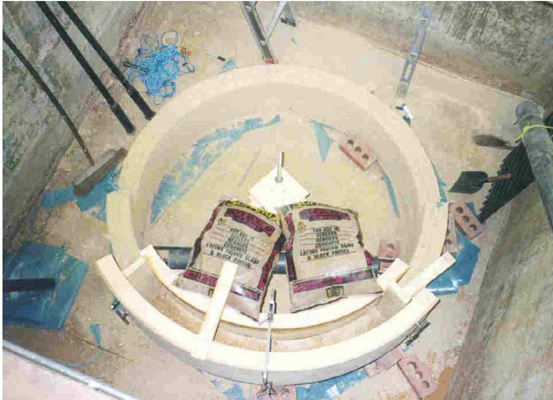
Figure 6 – Bird's eye view of the rammed earth tank under construction in the test pit at the University
