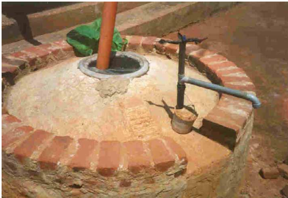
Figure 3 - A completed PBG tank showing inlet pipe and handpump for extracting water
