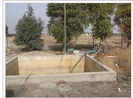
Effluent storage tank from where treated effluent (after constructed wetland) is pumped away for irrigation, Haran-Al-Awamied, Syria
