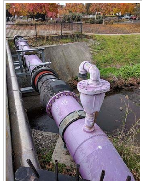
A lavender-colored pipeline carrying nonpotable water.
