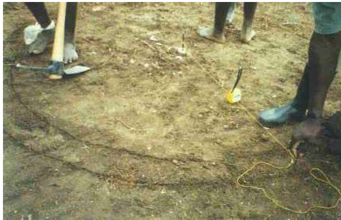
Figure 2 - Showing the cleared ground and the markings in place for the ring beam
