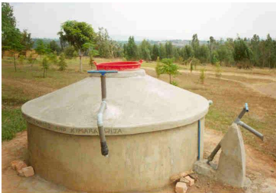
Figure 14 - Showing two types of handpump (DTU and Tamana), filter basin and externally rendered parapet wall, on this demonstration tank at Kyera Farm, Mbarara, Uganda. The guttering has not yet been fitted.
