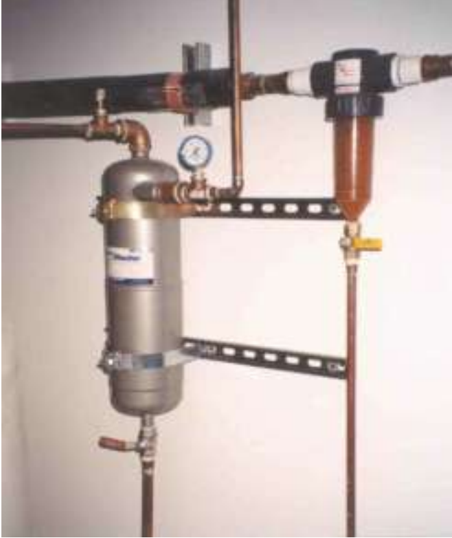
Sand filter and tank pre-filter
