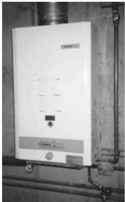
Tankless instantaneous hot water heater
