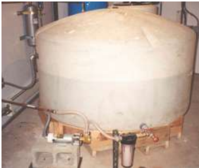
500-gallon water storage tank
