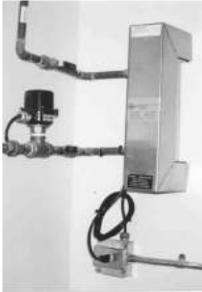
Flow switch and ultraviolet water purifier
