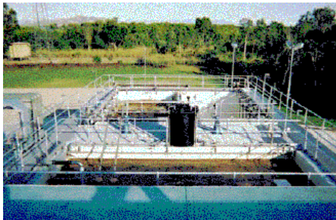
Fig. 25 Membrane bioreactor plant (Aquatec-Maxcon, 2004b)
