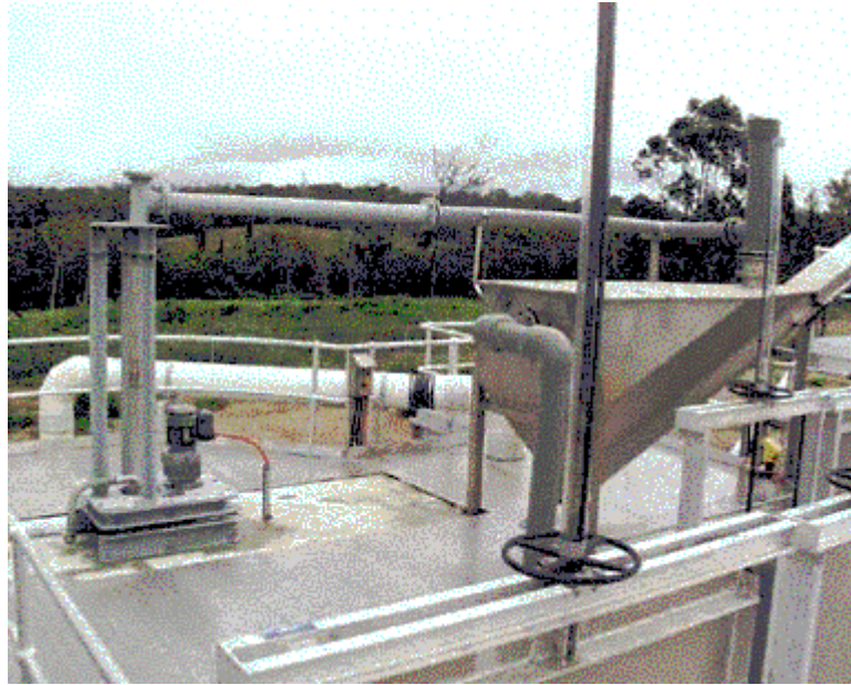
Fig. 6 Grit Removal (Aquatec-Maxcon, 2004a)
