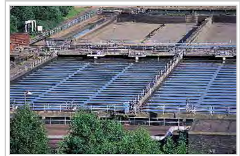
Sand filter used for water treatment
