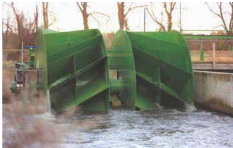
Fig. 18 (above) Photo of Staudruckmaschine installed (45)
