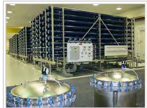
Reverse osmosis production train, North Cape Coral Reverse Osmosis Plant
