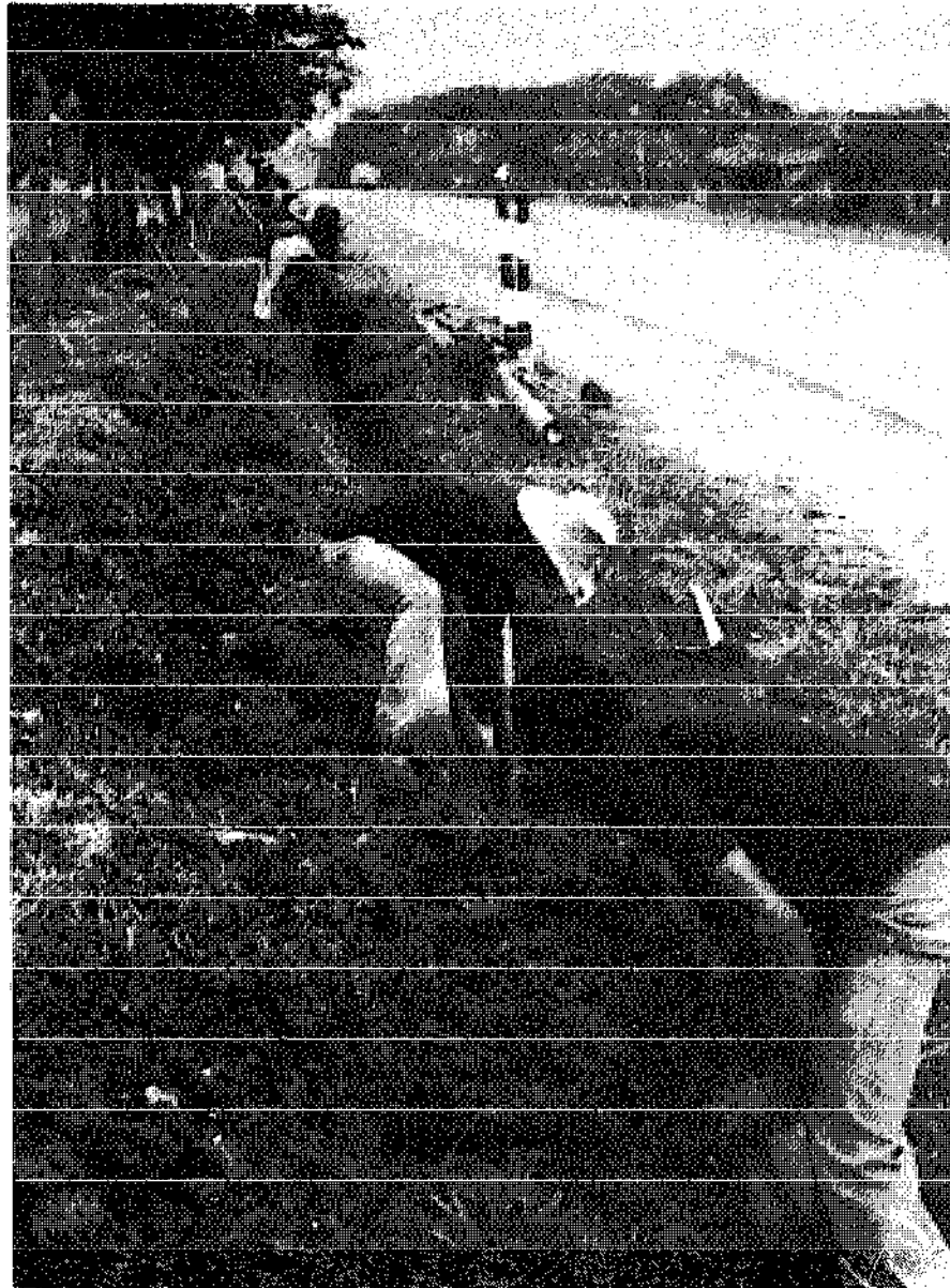
Figure 2.4: Community support in digging trenches for the distribution network, Alto de los Idolos, Colombia
