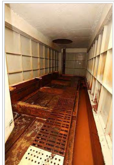
Empty aeration tank for iron precipitation
