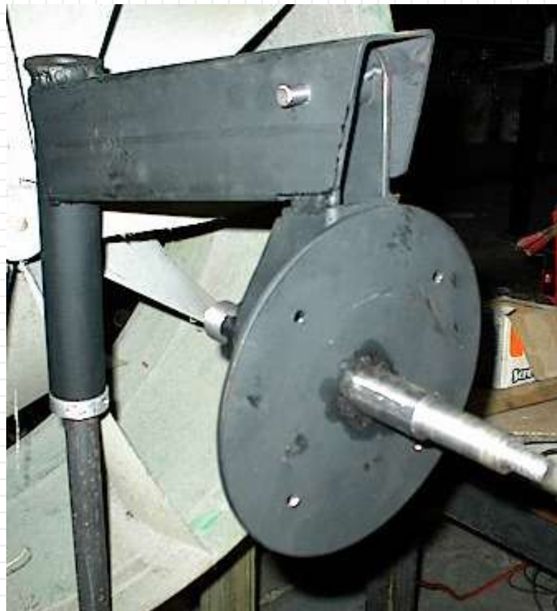
Below is a shot of the stator installed and the wiring almost completed.
