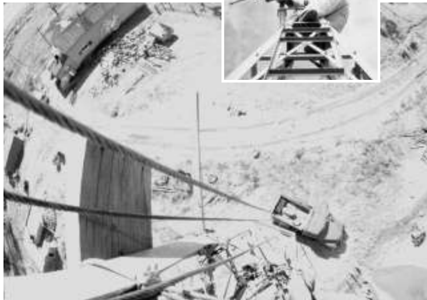
(Right) A Jacobs windplant is wrestled into place atop a tower. (Below) The view from 60 feet up
