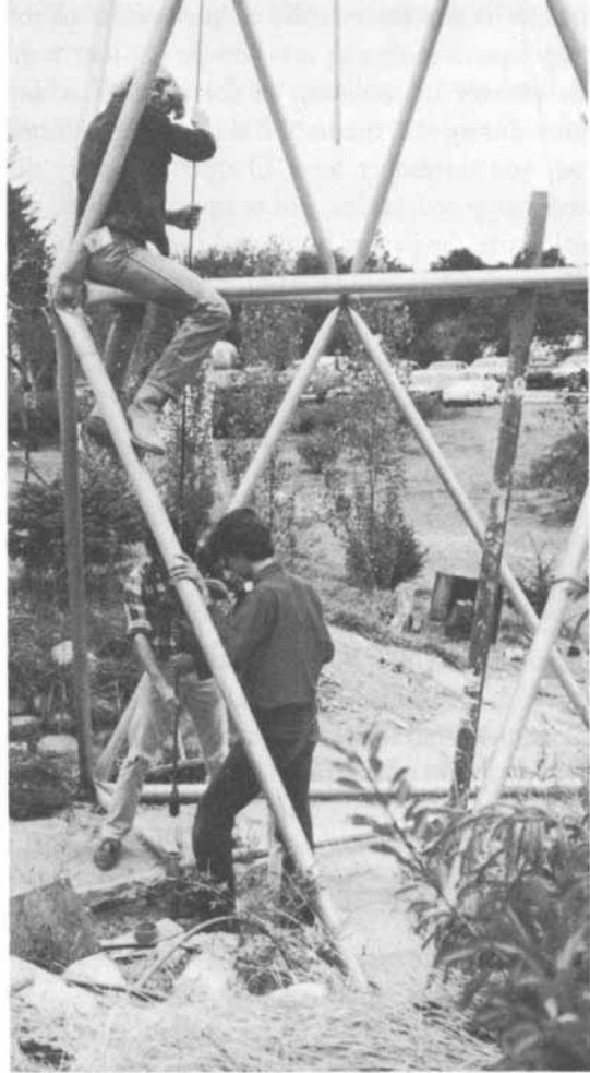
Figure 5.7. Station an elevated person above the well when lowering the pump rod.
