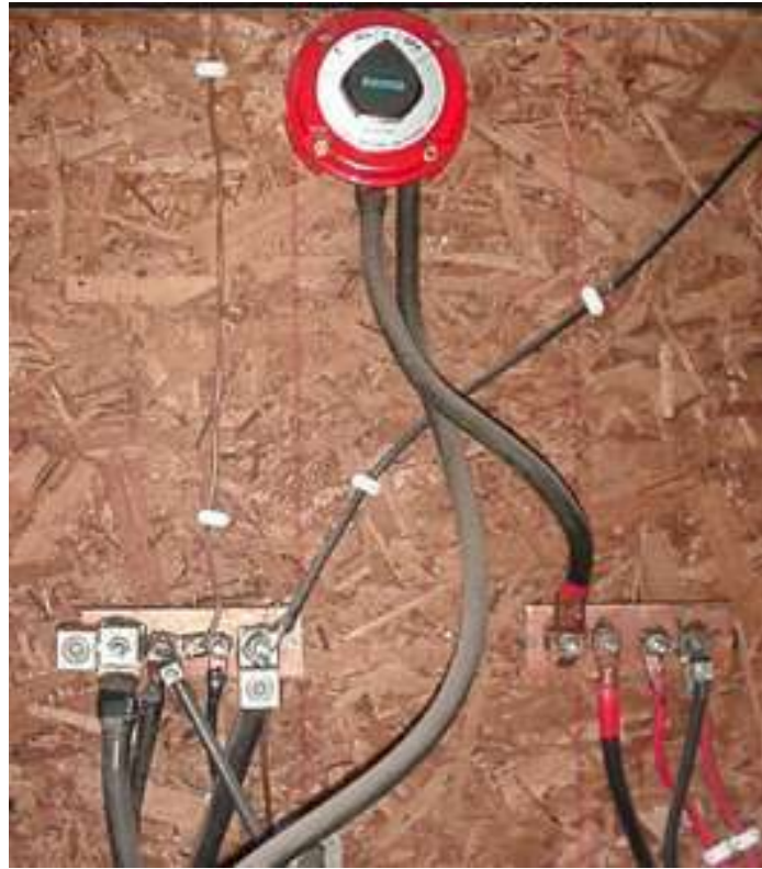
My buss bars and main power switch
