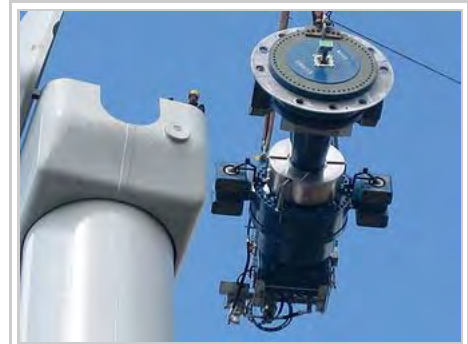
Components of a horizontal axis wind turbine (gearbox, rotor shaft and brake assembly) being lifted into position
