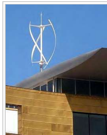
A small Quietrevolution QR5 Gorlov type vertical axis wind turbine in Bristol, England. Measuring 3 m in diameter and 5 m high, it has a nameplate rating of 6.5 kW to the grid.
