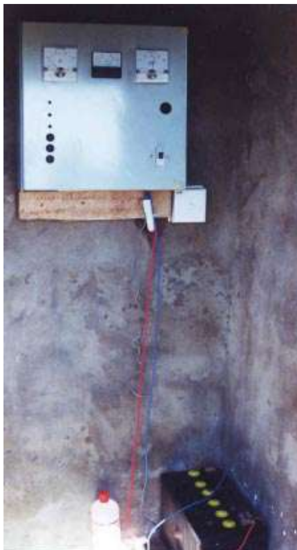
Photo 8: Wind generator control cabinet and car battery. (Simon Dunnett, Sri Lanka)
