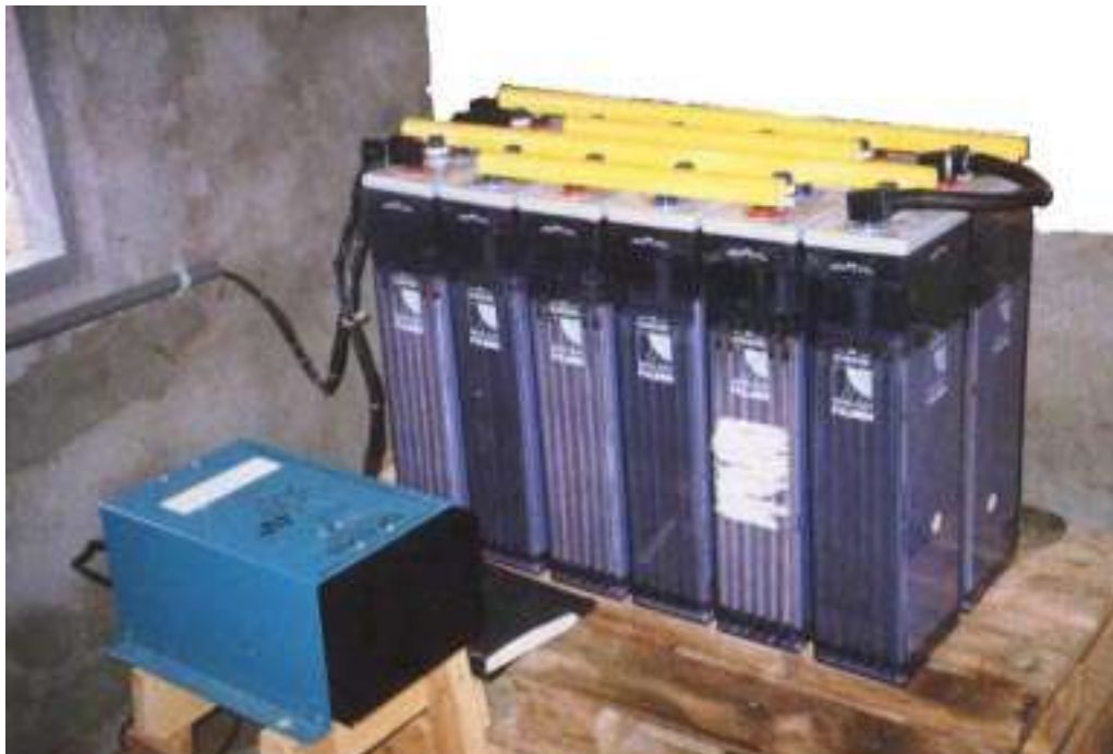
Photo 13: Deep cycle' Solar' battery in Sri Lanka. Twelve 2 volt cells with 900 Ah capacity are connected to make one 24 volt battery with 900 Ah capacity. Height is 700mm. On the left is an inverter. ( Hugh Piggott )
